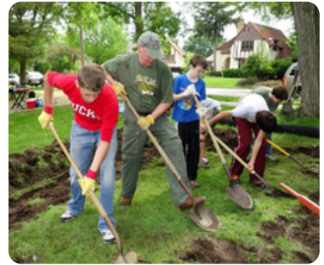
Installation of the lower rain garden at Thoreau Elementary School. Photo by David H. Thompson
